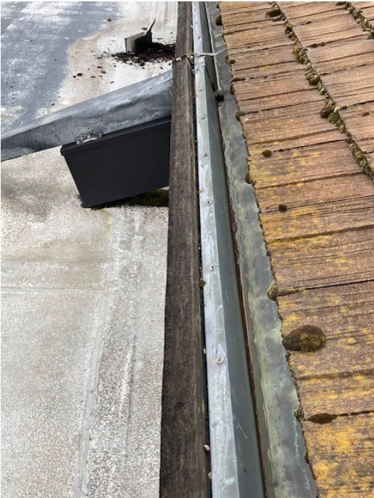
6. Gutter above South side (over offices) above flat roof.
